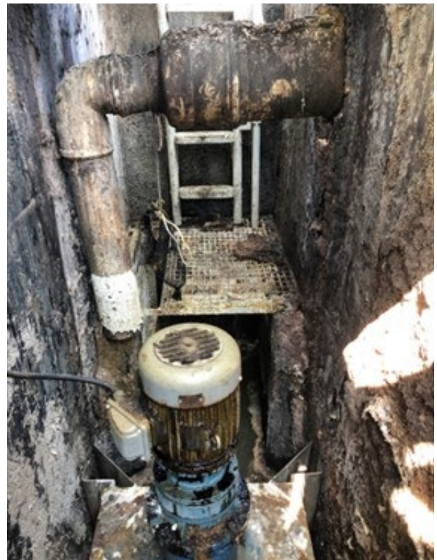
LINE 59 STATE ROAD PUMP STATION $400,000
